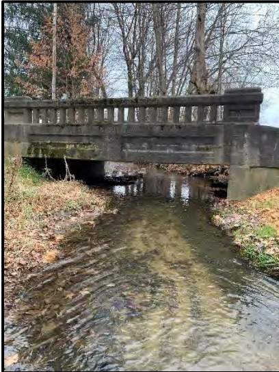
Photo 23: 11/24/2020 – STREAM-1, sample point location, facing north at Campbell Road.
